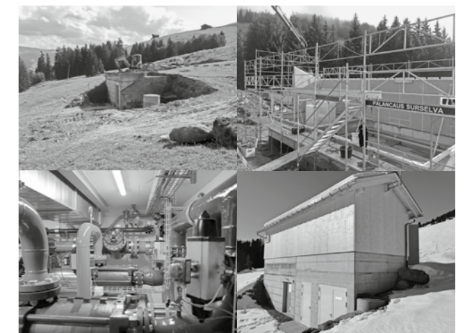
Neue Pumpstation PS100 in Gneida
